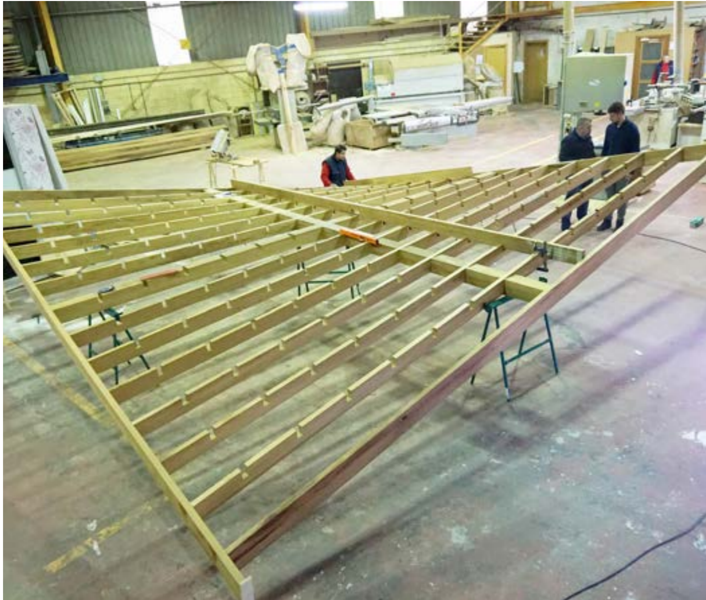
Marquesina no taller © Ezcurra e Ouzande Marquesina en taller © Ezcurra e Ouzande Canopy under construction © Ezcurra e Ouzande
